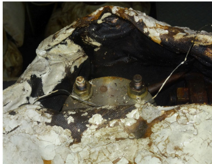
Picture 26 - insulation wetted through oil & damaged
