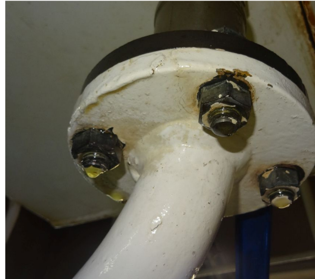
Picture 13 - everywhere small oil leakages
