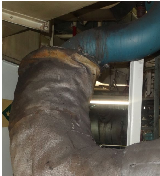
Picture 21 - missing insulation
