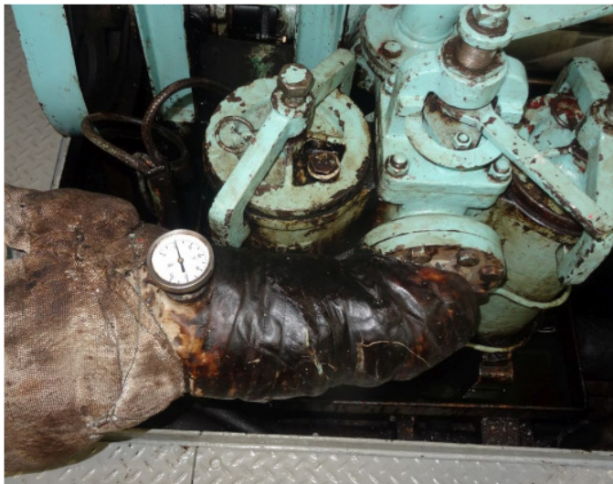
Picture 25 - insulation wetted through oil & damaged
