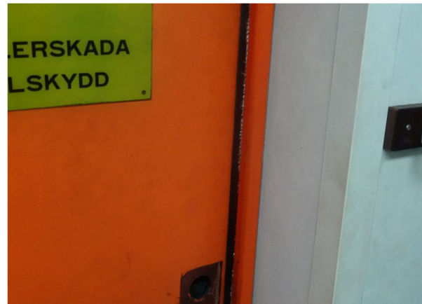
Picture 37 - door not closing, missing lock
