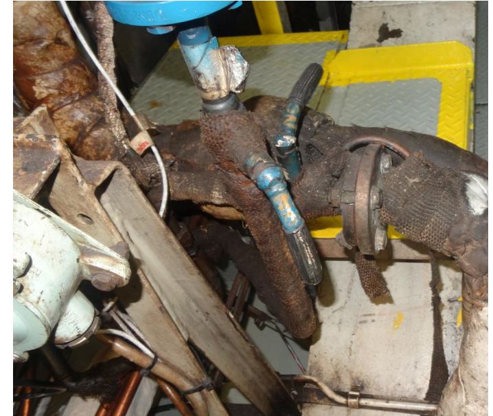
Picture 24 - insulation wetted through oil & damaged
