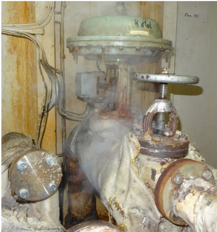
Picture 34 - steam leakage
