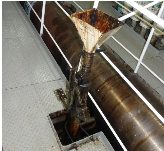
Picture 30 - ...which kept sounding pipes open
