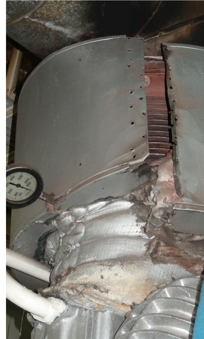
Picture 22 - damaged insulation
