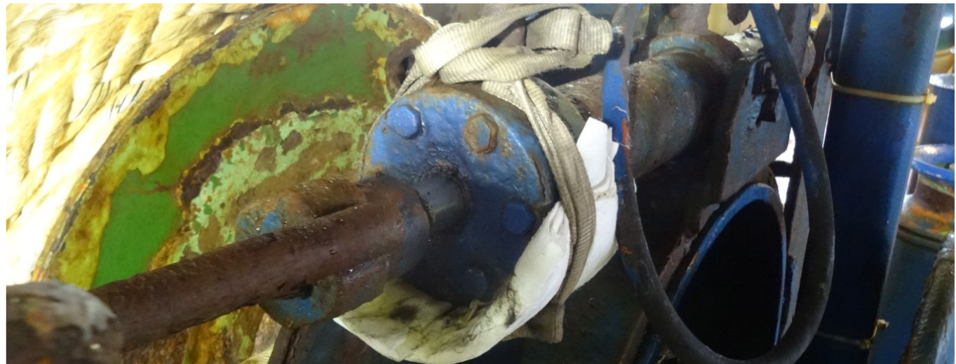
Picture 5 - known oil leakages on mooring winches found "temporary" repaired
