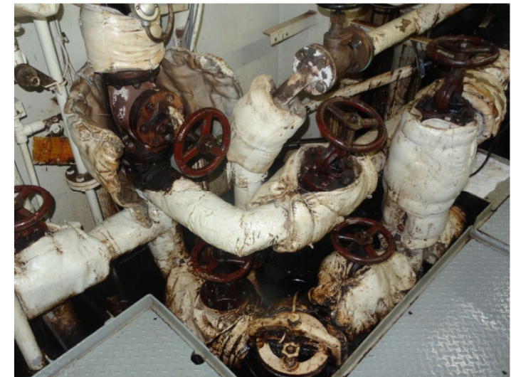
Picture 27 - insulation displaced
