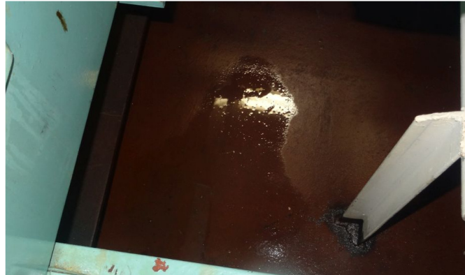
Picture 19 - fuel leakage on emergency generator
