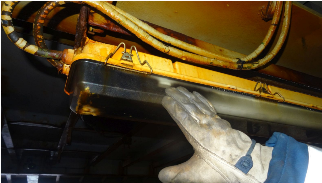
Picture 6 - when switching on, the lights on pilot station caught fire...
