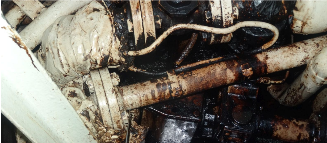
Picture 23 - insulation wetted through oil, insulation partly missing and HFO spill
